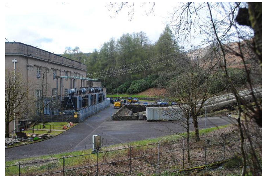
Transformers located at rear of the power station
