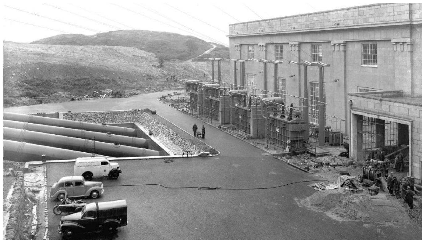
View of the rear of Sloy Power station including view of area to the north of the site cleared for construction activities. Photograph taken circa 1950.
