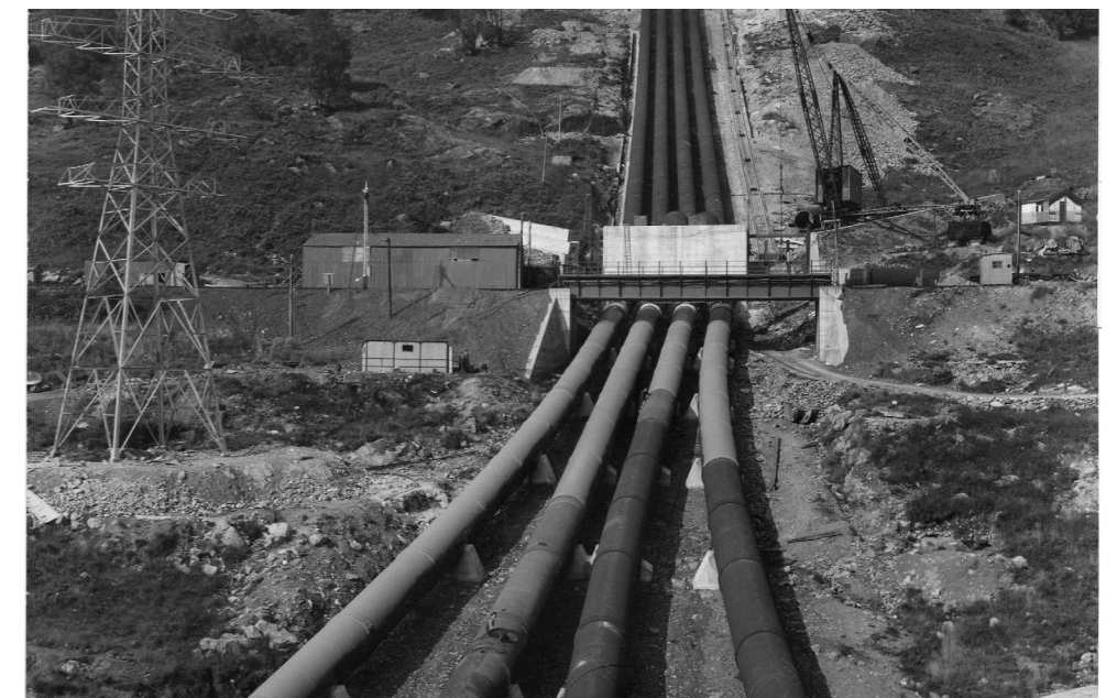
Sloy Penstocks; Image Credit: SSER
