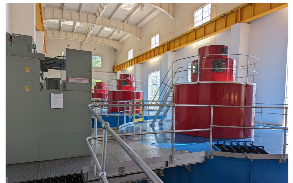
Sloy Turbine Hall; Image Credit: Page\Park Architects
