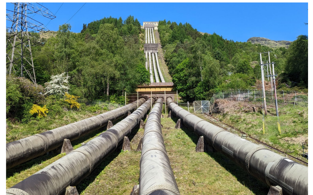
Sloy Penstocks; Image Credit: Page\Park Architects
