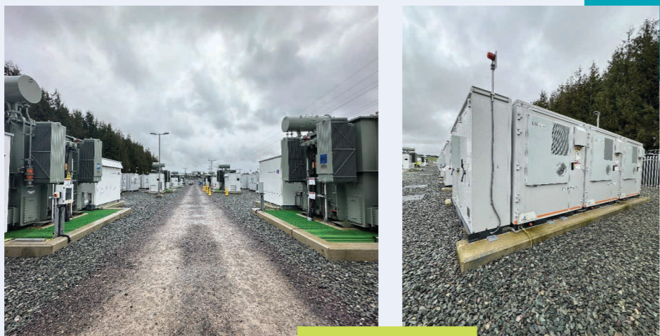
Image 1 and Image 2: The SSE Salisbury Battery Storage project in Wiltshire, England. A project similar in design to the proposed Mullafarry BESS.
