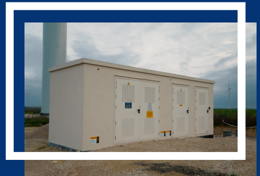
Delivery substation: place where all turbines are connected before electricity is forwarded within a single cable to Vertus's outgoing substation to then be injected into national grid.
